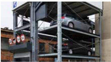
Maintain automated car parking systems
