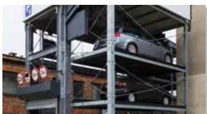
Maintain automated car parking systems
